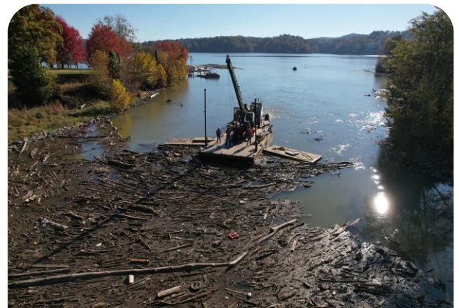
Waterway Debris Removal
