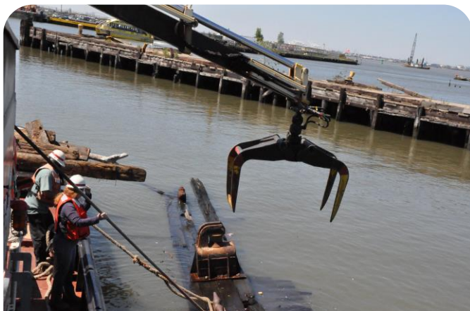
Waterway Debris Removal
