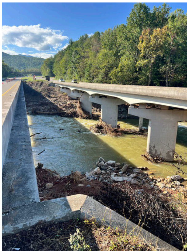
Improved drainage canal choked with vegetative debris — the typical condition WDS will restore.
